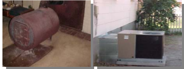
Replacing inefficient wood burning heaters with central heating units is an example of how the City is addressing the need to improve housing quality.
